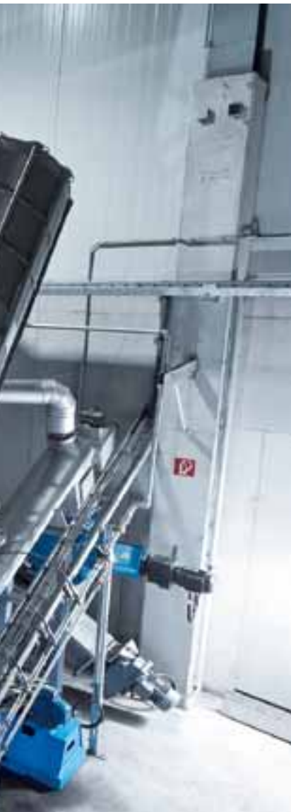
Pilot plant for the torrefaction of biomass: improvement of biomass fuel properties and savings in CO 2 .
